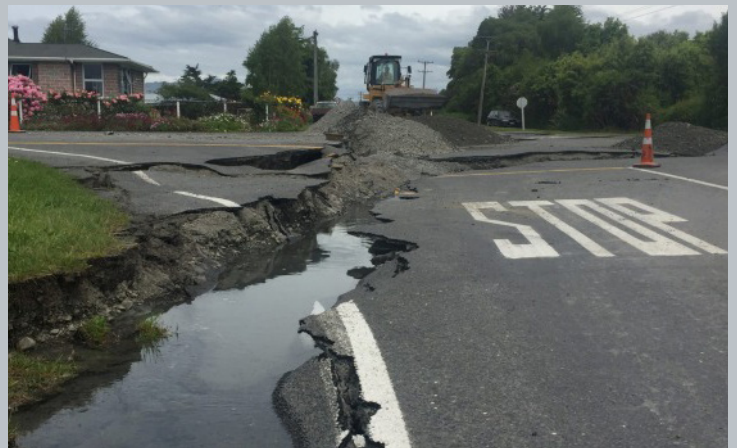
The huge quake ripped up roads throughout the town main town.
